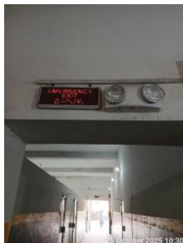
Emergency exit sign & light-2.jpg
